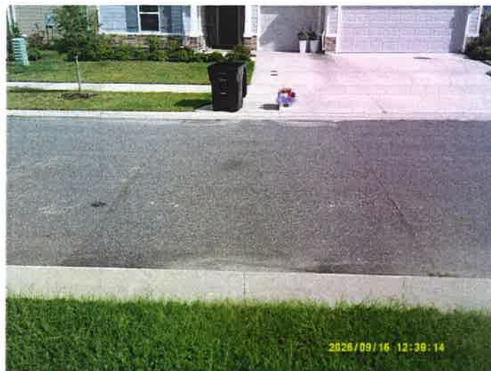
Figure 3 – Pavement Distress – Area 2
