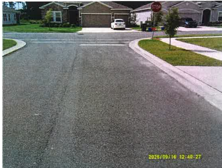
Figure 4 – Pavement Distress – Area 3
