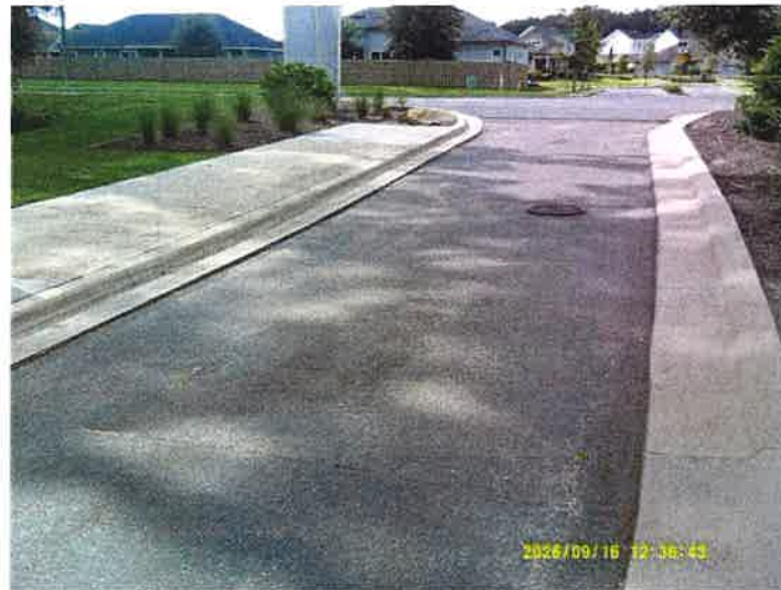
Figure 2 – Pavement Distress – Area 1
